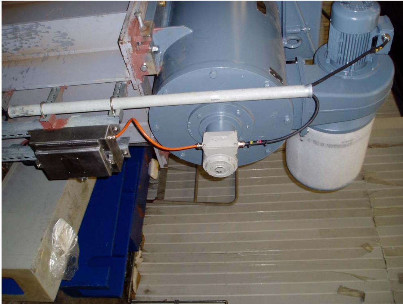
UNIT-ONE basic unit installed on STS cranes Eurogate Hamburg
