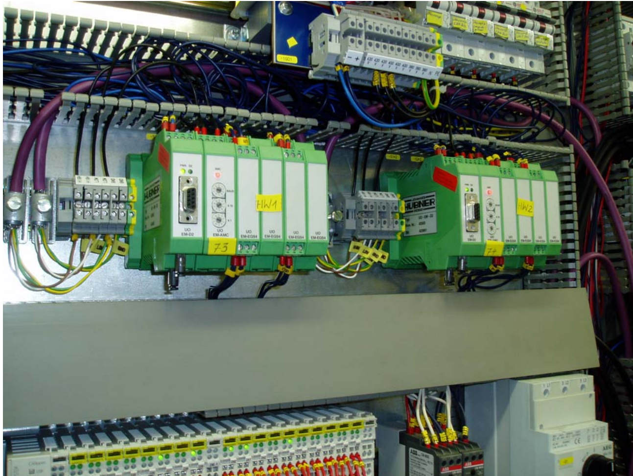
UNIT-ONE electronic function moduls installed on STS cranes Eurogate Hamburg
