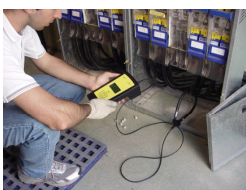
Cable identification in the LV output of an MV/LV transformer using the IC1G receiver (RX)
